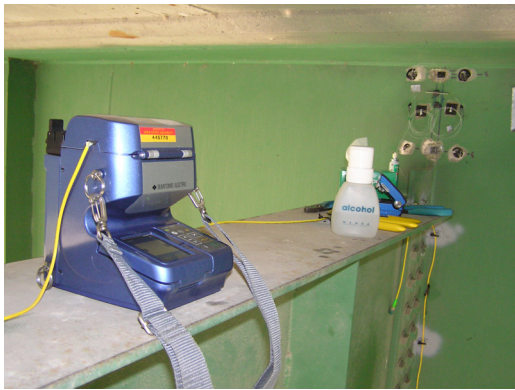
c. Fiber optic equipment used for fusion splicing
