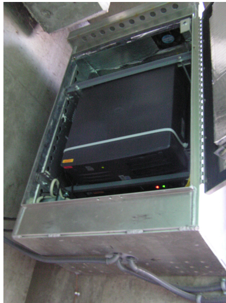
Figure 4.5. Temperature-controlled cabinet containing the data management and collection equipment at the US30 bridge.
