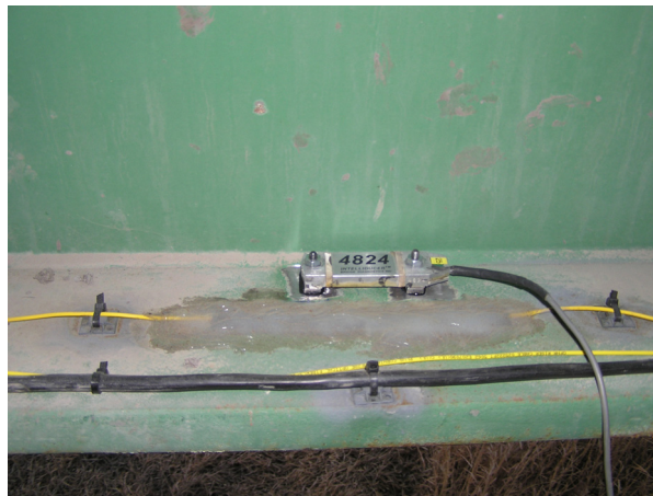
Figure 4.9. Typical placement of a BDI sensor relative to a FOS during in-service validation testing.
